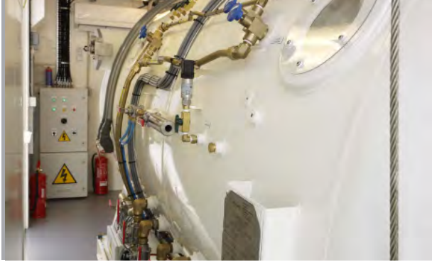
A 1600 mm decompression chamber inside a 20 ft. container.
