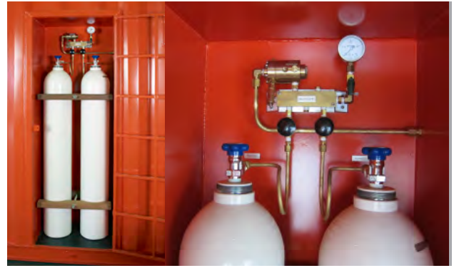
Gas supply two oxygen cylinders and reducers.
